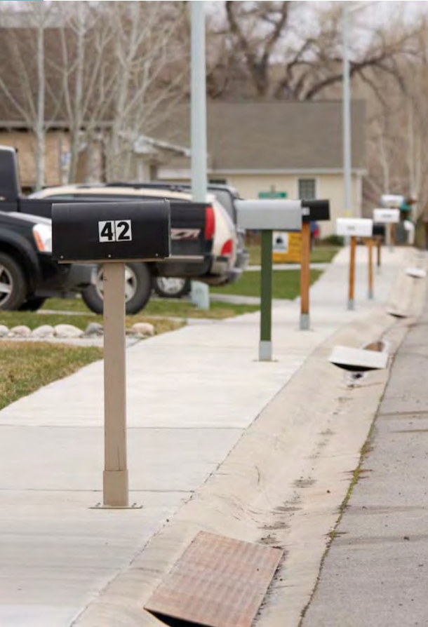
Generally the utility infrastructure is in good condition. However, while some areas have formal storm drainage, others lack the necessary infrastructure.
