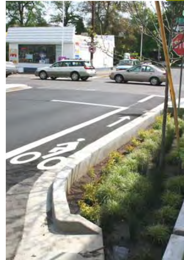
Utility upgrades may include new sustainable stormwater management techniques, including vegetated planters.
